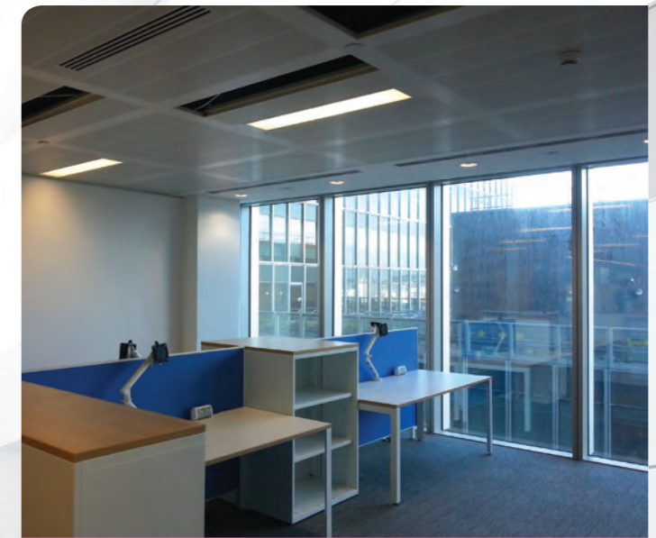
The lights are on in this office despite the abundant natural light. It is important to integrate lighting controls with daylight availability, so that artificial lighting is dimmed or switched off when there is sufficient daylighting
