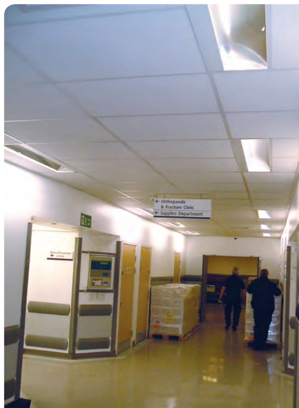
Lighting was assessed across the hospital, including here, where ceiling lights in an asymmetric lighting system direct light onto walls
